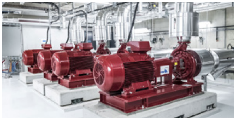
The Thassalia project in Marseille (France) is a seawater district heating and cooling system that services 600,000 m 2 of buildings.
